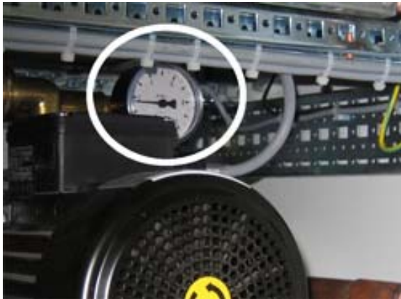
Fig. 3: Manometer of cooling circuit
